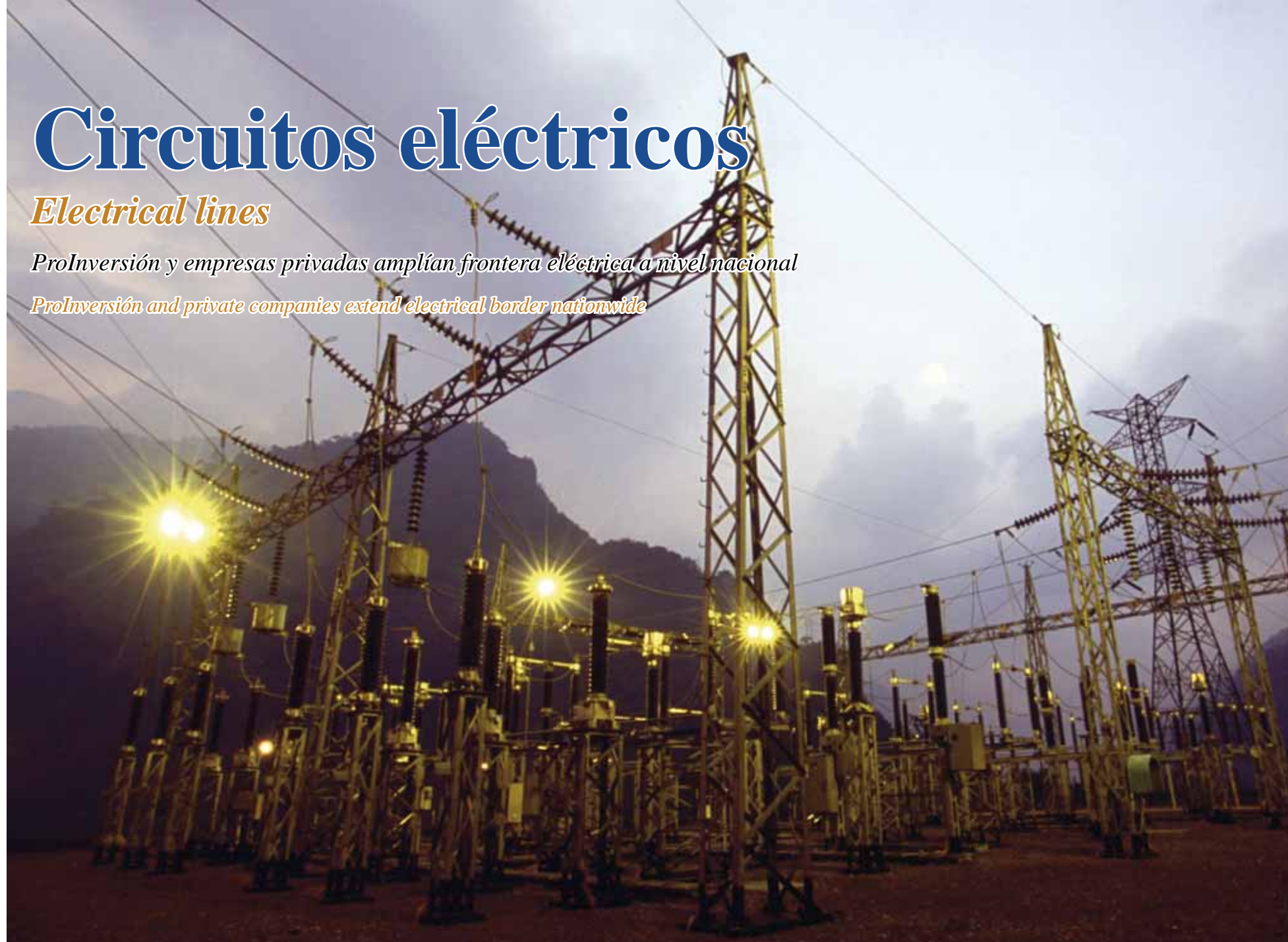
La electricidad es imprescindible para el desarrollo de un país. The electricity is essential for the development of a country.
